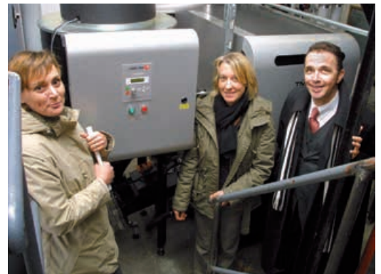
Cornelia Peer (owner of HTEC, Kamp-Lintfort), project leader Miriam Kramp and mayor Dr. Landscheidt (f.l.t.r.) inspect "Kinderhaus Kunterbunt" nursery's new biomass heating system.
